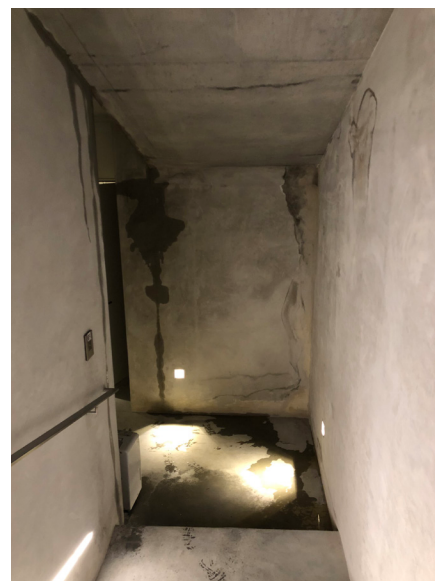
Fig 3 -- Before: stubborn water seepage was exacerbated by near record rainfall during construction. [photo courtesy Sheila Lee Davies]
